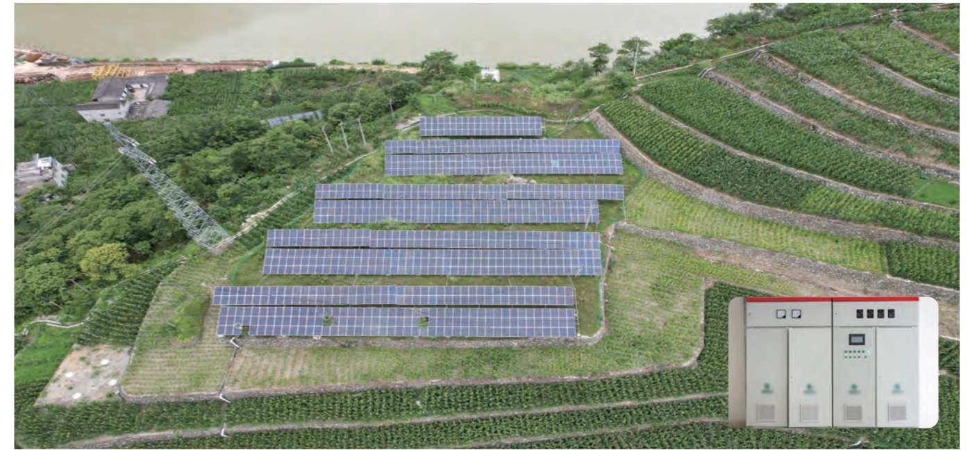
246kW Controllers: 2*PDS33-4T075 + 2*PDS33-4T015 Location: Sichuan Province, China
