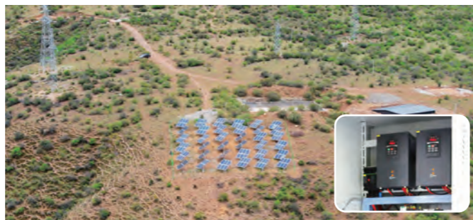
95kW Controllers: 2*PDS33-4T037 Location: Sichuan Province, China
