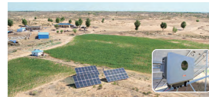
18.9kW Controllers: 3*PDS51-4T004-E Location: Inner Mongolia, China
